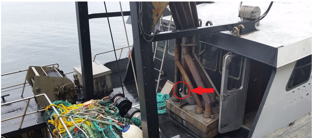
Figure 2 - Problematic “float-free” EPIRB installations
