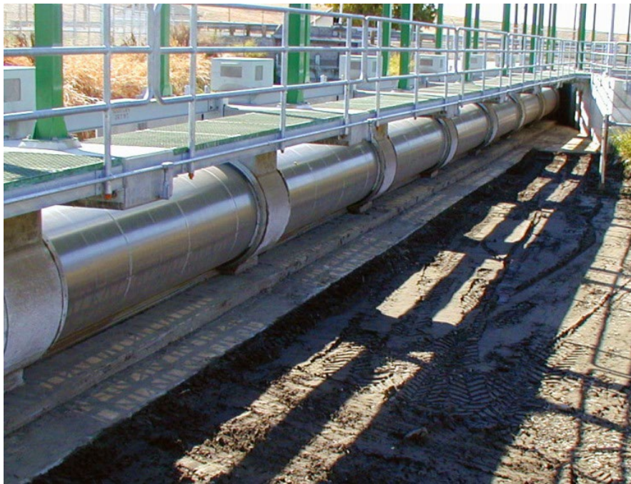
Figure 8-8 Medium-sized rotary drum screen at the Burlingame Diversion located on the Walla Walla River near Walla Walla, Washington
