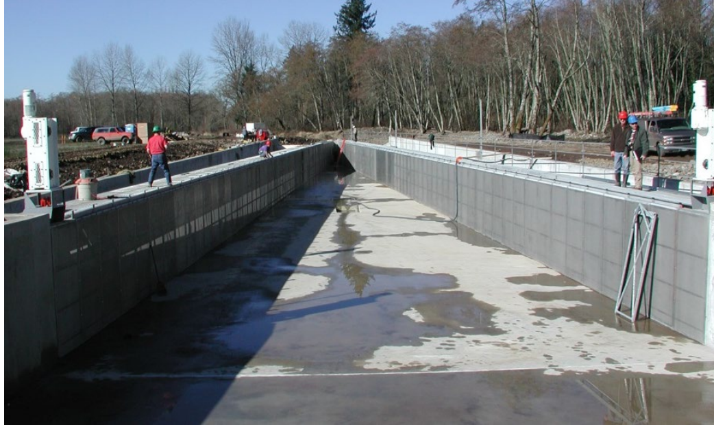
Figure 8-5 Vertical plate screen facility under construction in a diversion canal located on the Santiam River near Stayton, Oregon
