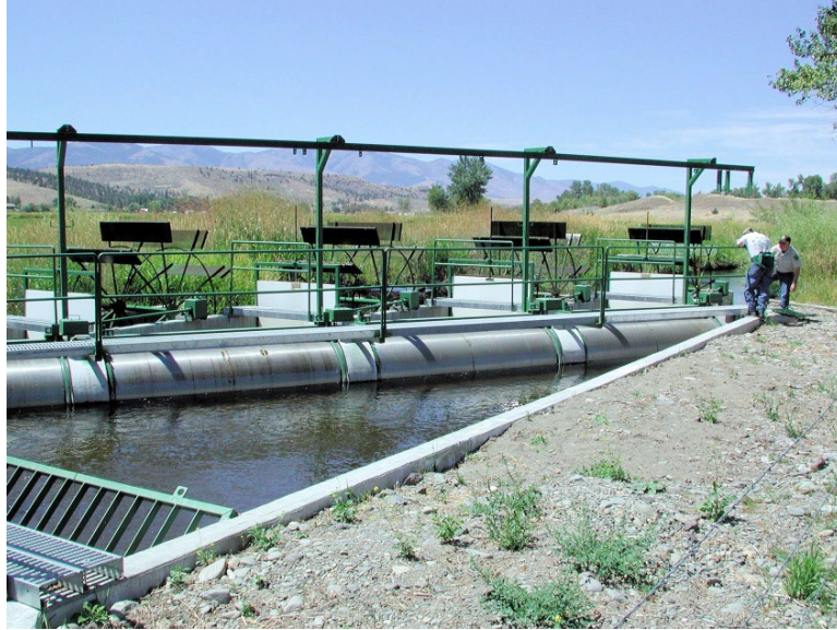
Figure 8-9 Rotary drum screens installed in a water diversion canal and operated (i.e., powered) by paddle wheels
