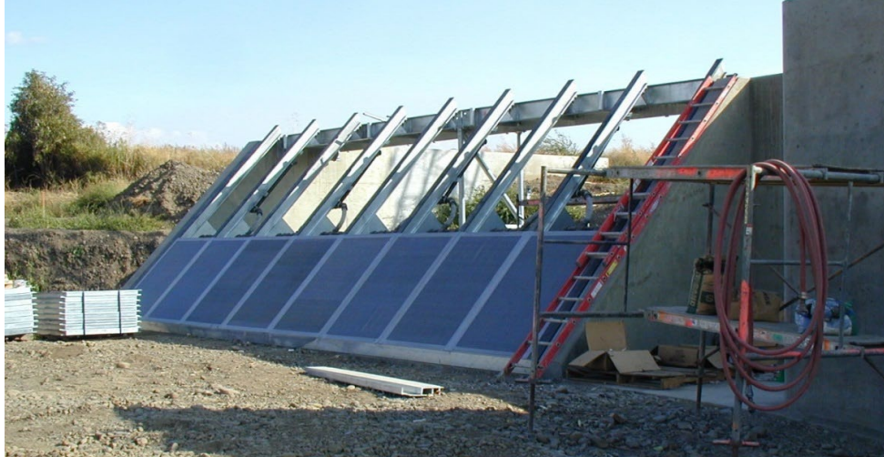
Figure 8-2 Bankline screens at the Garden City-Lowden 2 diversion on the Walla Walla River near Touchet, Washington, under construction
