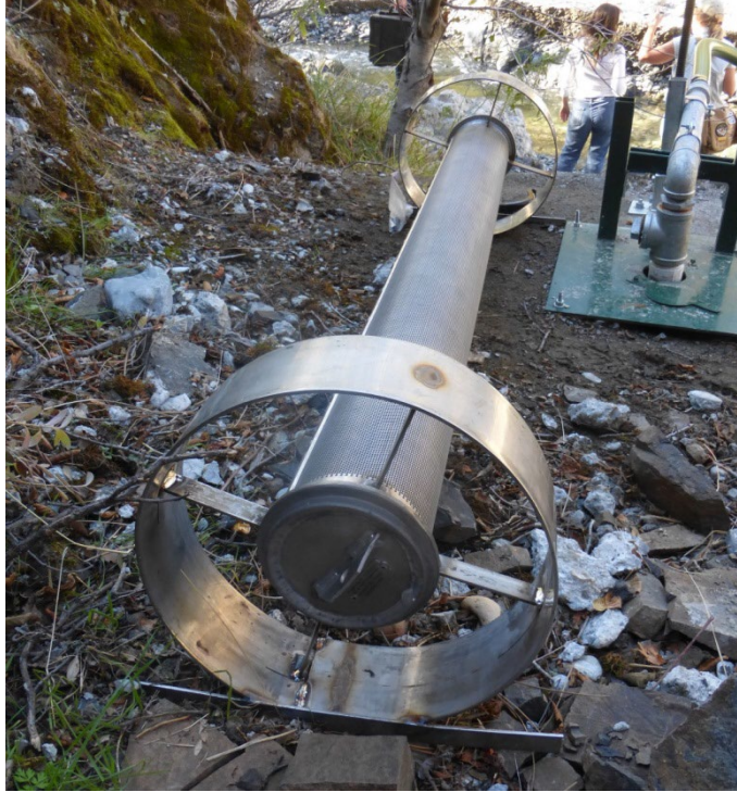
Figure 8-10 Typical end-of-pipe screen equipped with “wagon wheels” to elevate the screen off the stream bottom
