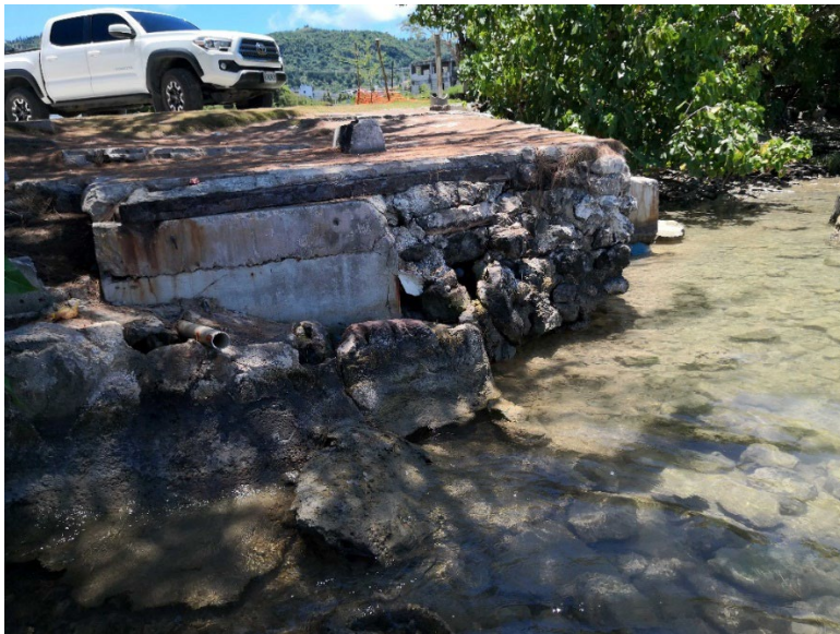
Figure E-4. Cement foundation and cemented seawall to be demolished. Credit: CNMI DLNR 2021.
